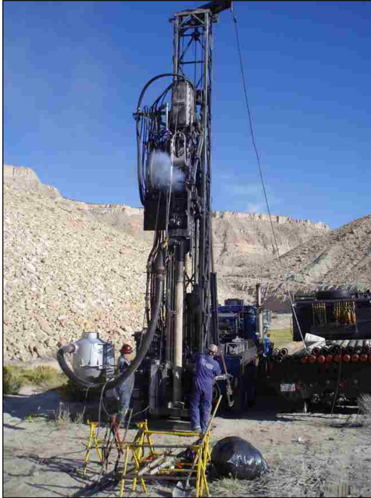
Figure 2-1. Becker Hammer Rig used at Millsite Dam in 2009, view looking north along the downstream toe of the dam.
