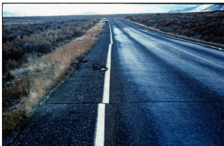
Figure 6-3. Photograph showing lateral displacement of Highway 93 near the 1985 Whiskey Springs investigation site (Youd et al. 1985).
