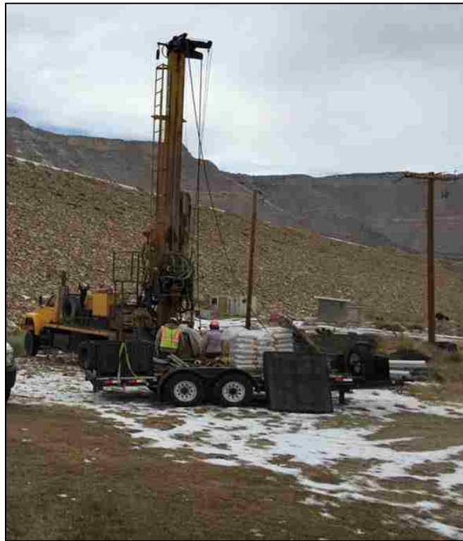
Figure 8-3. View of drill rig used at Millsite Dam looking north along the downstream toe of the dam, January 2015.
